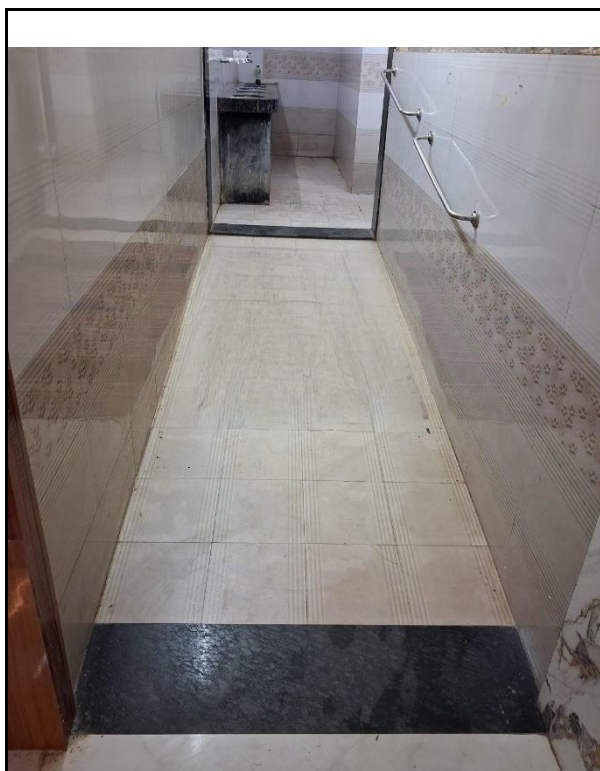
Rampway Entrance Toilet — Support Handrail
